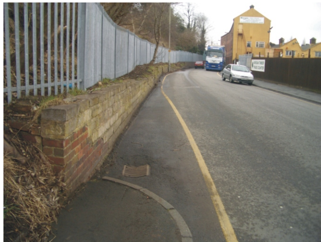
Photo 6.9 - Retaining wall of variable height and quality. End of footpath on west side of Park Lane.
