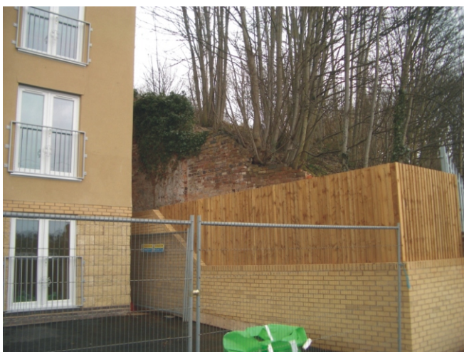
Photo 6.14 - High retaining wall adjacent to new apartments requires structural survey. Need to consider relationship with neighbouring sites.
