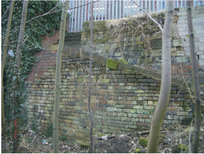
Photo 6.5 - Stepped access to industrial units on Park Street in disrepair
