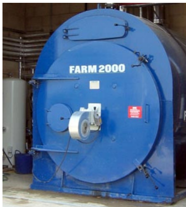
Figure 2 Big bale burner / boiler 13
