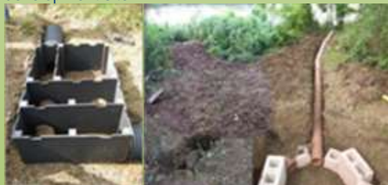
Artificial otter holt – internal construction (L) and external view during installation (R). Note: how the holt can be installed above or underground and integrated into soft-landscaping if adequately protected from disturbance.
