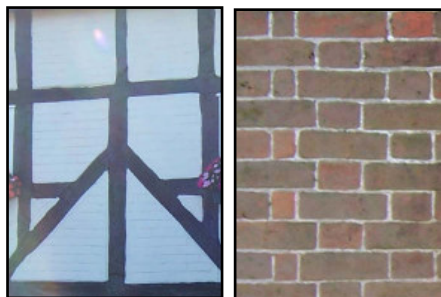
Example of materials used in the Area include timber framing with brick infill and brick
