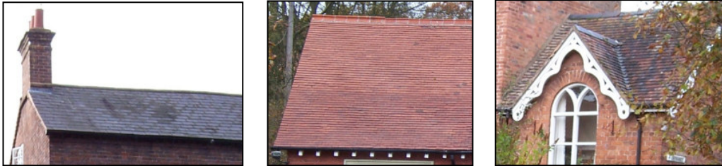
An example of the roofing materials and colours found within the Area
