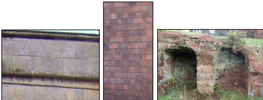
Examples of some of the different building materials used throughout the Area: sandstone ashlar; brick, sandstone
