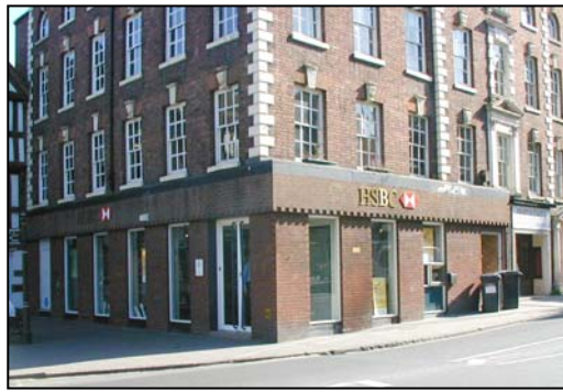
Unsympathetic alterations to the ground floor of HSBC in Load Street
