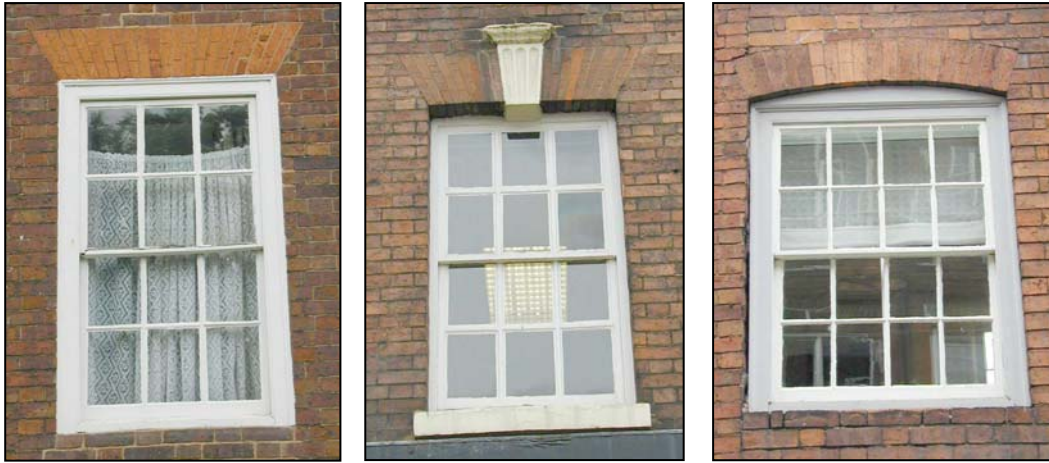
Close up of a front mounted sash window with gauged voussoirs (left) recessed sash window with gauged voussoirs, keystone and stone cill (middle) and front mounted sash window with segmental brick header (right). Note that each voussoir to the flat headed windows is individually gauged and of a finer grain and quality than the brickwork, and that front mounted windows have wide architraves
