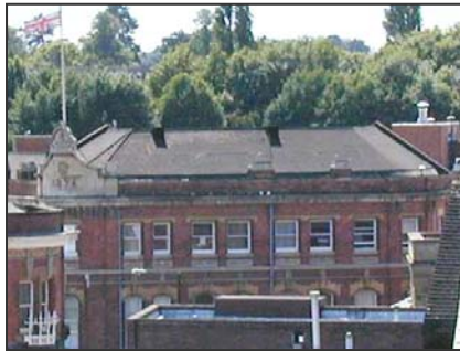
Principal roofs to Nos. 17 to 20, Vicar Street (top left), No. 66 Oxford Street (Barclays Bank) (top right) and Brinton's Offices (bottom)
